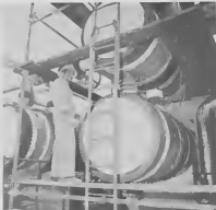
Federico Donata insulates heat exchanger covers at No. 5 Pipestill with block forms shaped into large circles. Note wires running criss-cross with nuts.
